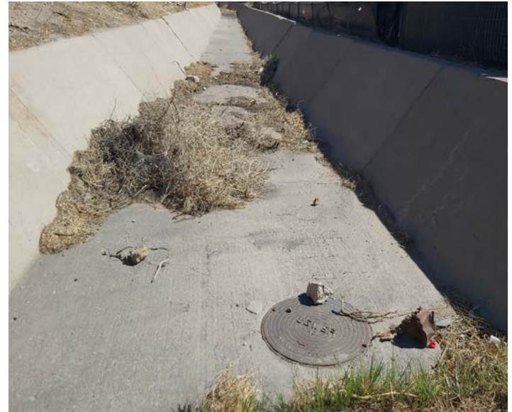
PHOTO NO. 4: General southeast view of existing concrete channel conditions and manhole.
