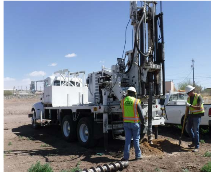
PHOTO NO. 24: General view of subsurface drilling operations at vertical boring B-10.
