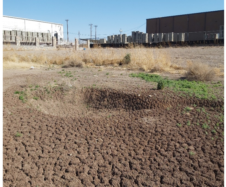
PHOTO NO. 14: General southeast view of existing ponding area conditions at vertical boring B-10.
