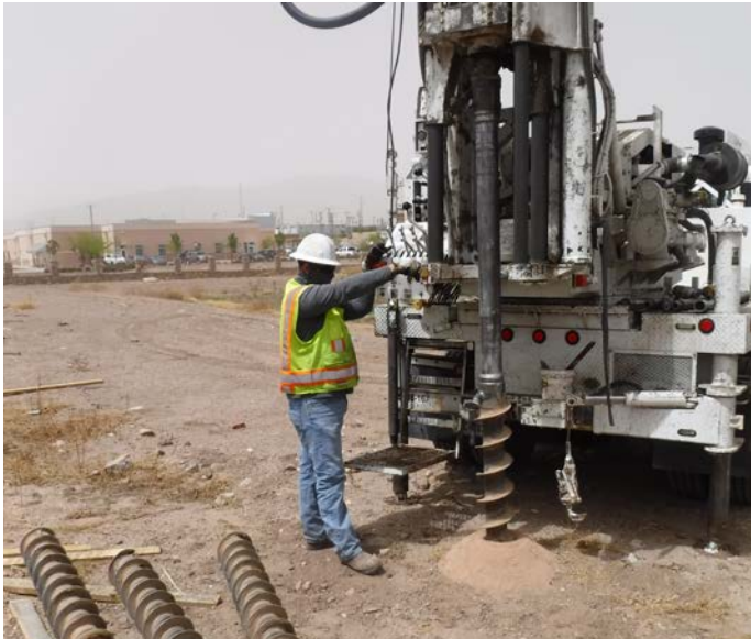
PHOTO NO. 23: General view of subsurface drilling operations at vertical boring B-9.
