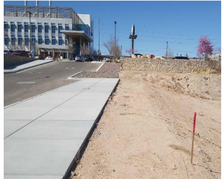
PHOTO NO. 8: General north view of box culvert route and existing conditions at vertical boring B-4.
