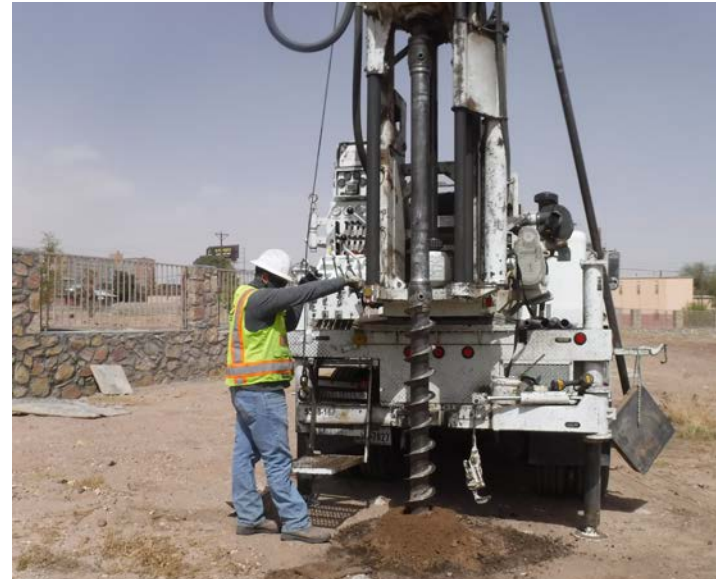
PHOTO NO. 20: General view of subsurface drilling operations at vertical boring B-5.
