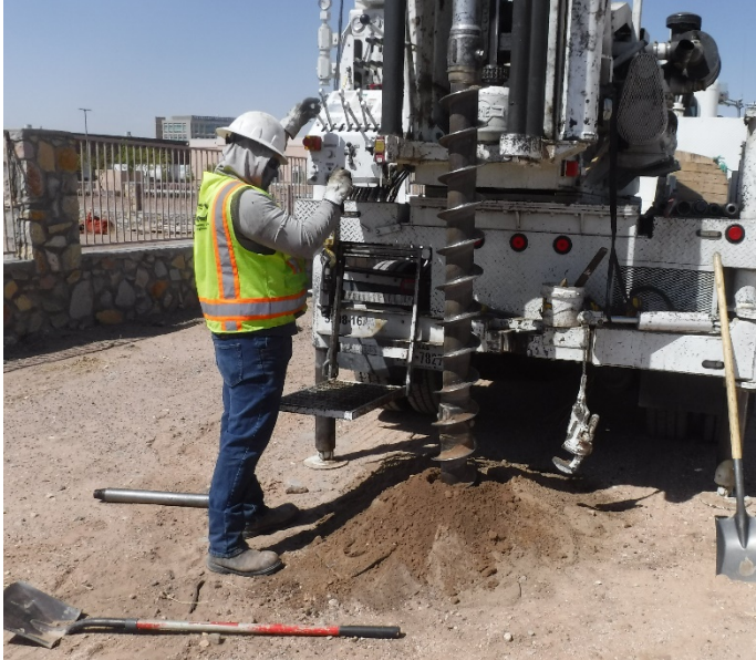
PHOTO NO. 21 General view of subsurface drilling operations at vertical boring B-6.
