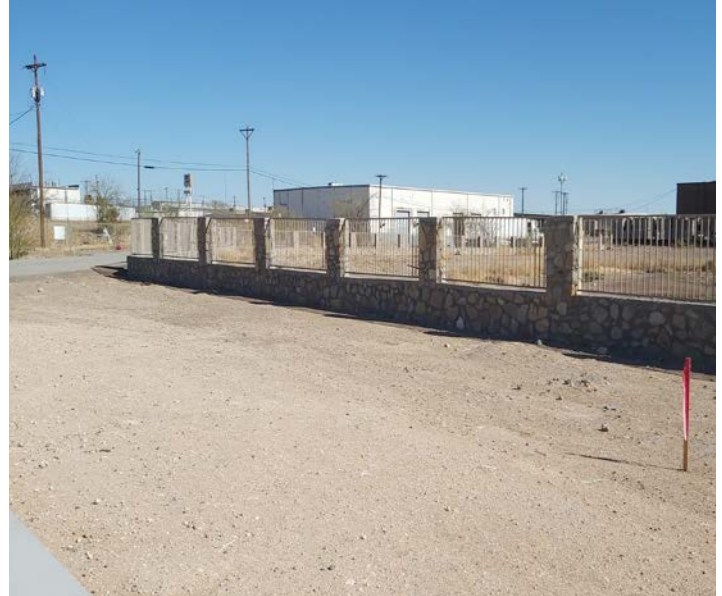
PHOTO NO. 10: General southeast view of box culvert route and existing conditions at vertical boring B-6.
