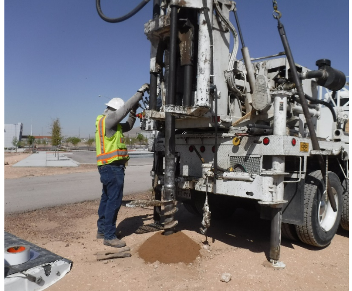
PHOTO NO. 22: General view of subsurface drilling operations at vertical boring B-7.
