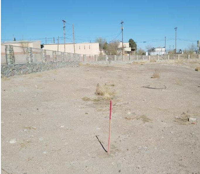
PHOTO NO. 9 General east view of box culvert route and existing conditions at vertical boring B-5.
